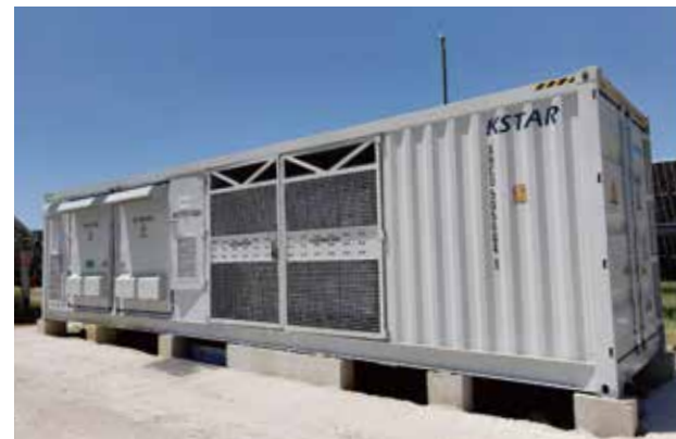
03 Utility Project in Spain 10MW PV Plant
