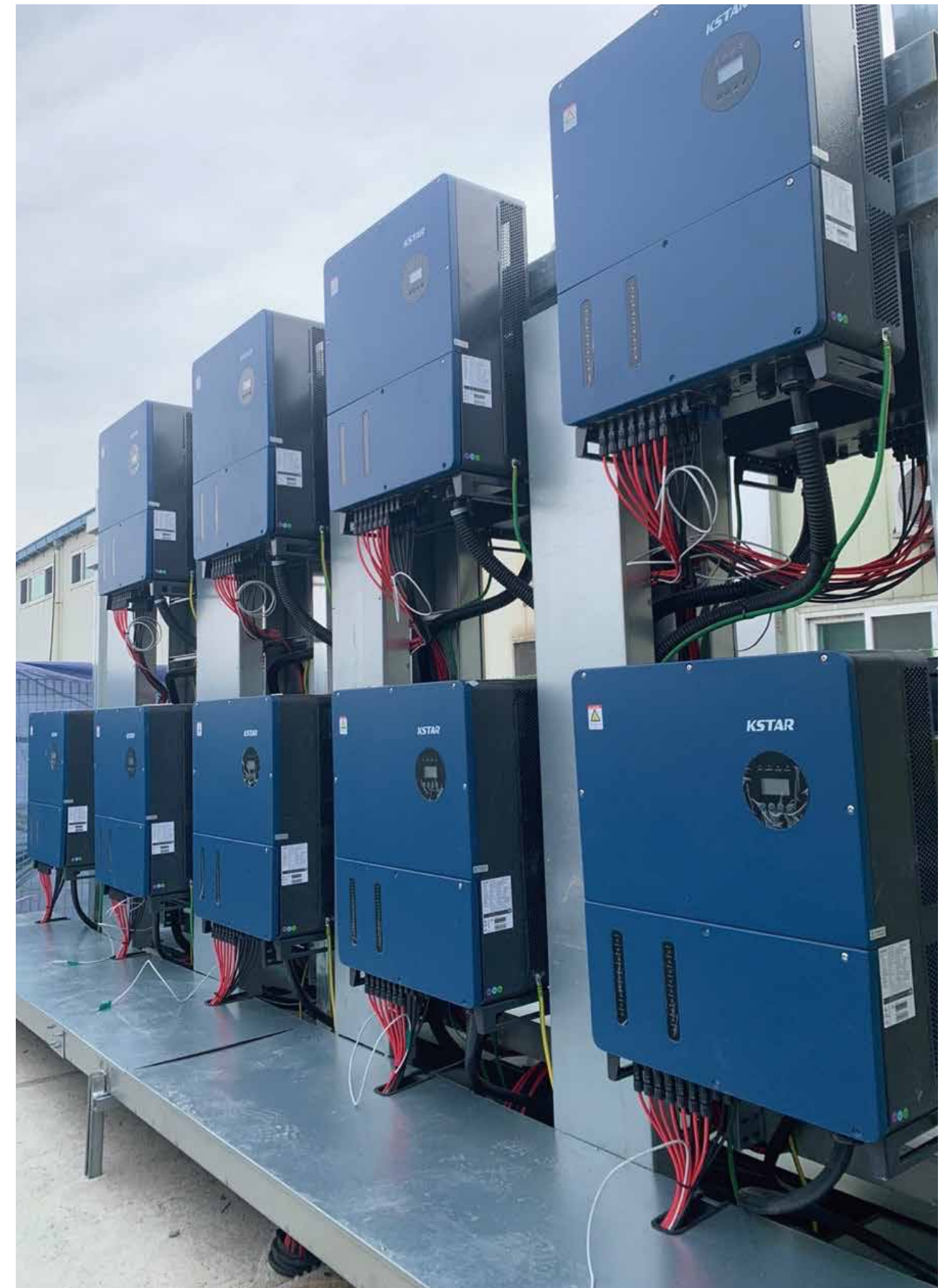
11 C&I Project in Daejeon 1MW, KSG-60K-A
