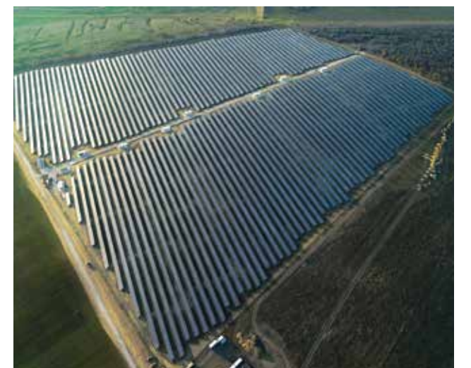
08 Utility Project in Ukraine 15MW PV Plant
