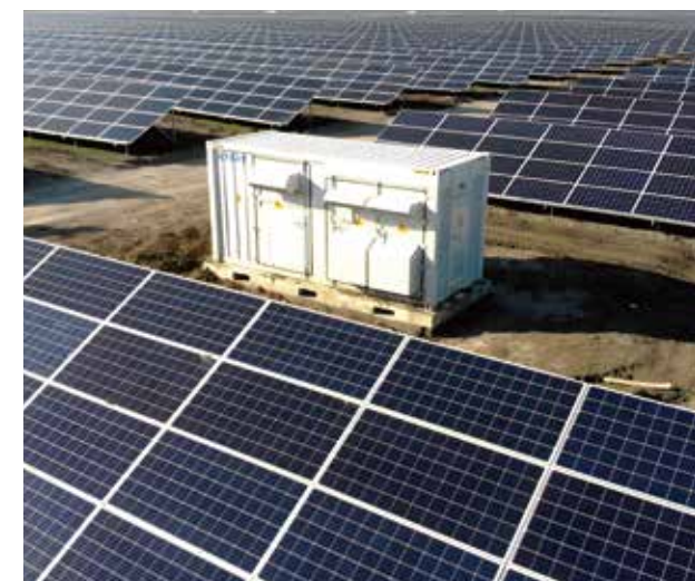
07 Utility Project in Ukraine 200MW PV Plant
