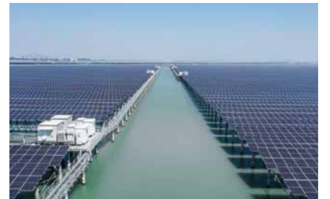
06 Utility Project in Zhejiang 550MW Watersurface PV Plant
